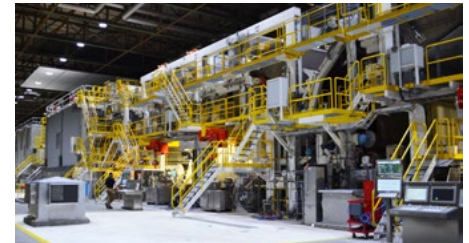
Paper Machine 1 at Somerset Mill.
